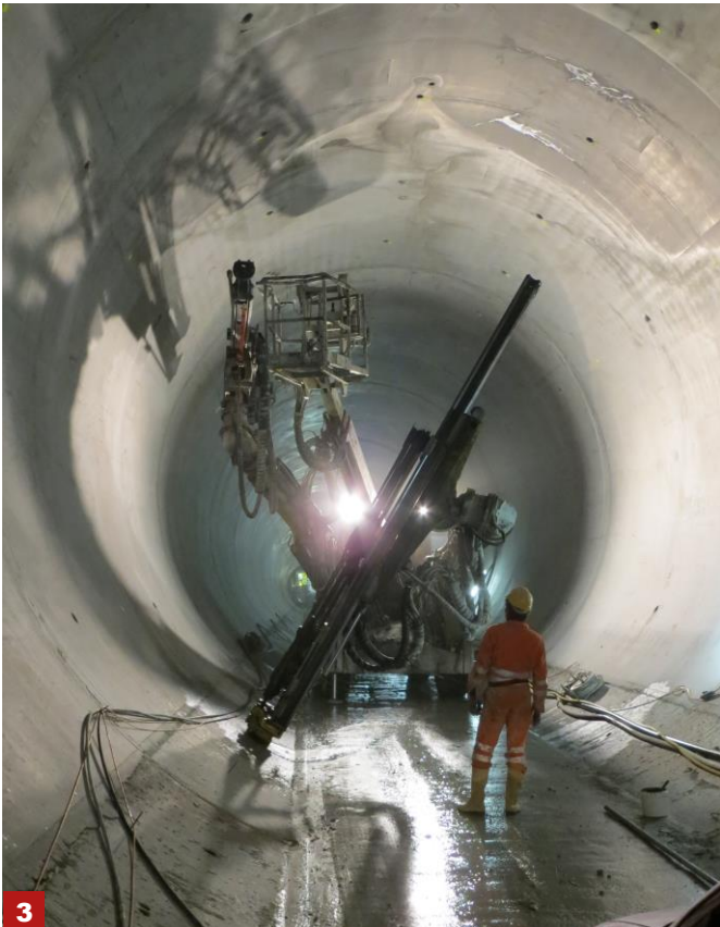
Front page: Bore holes for bulkhead grouting 1. Bulkhead grouting system diagram 2. Grout container (6 pumps) and mixing plant 3. Bore holes for contact grouting
